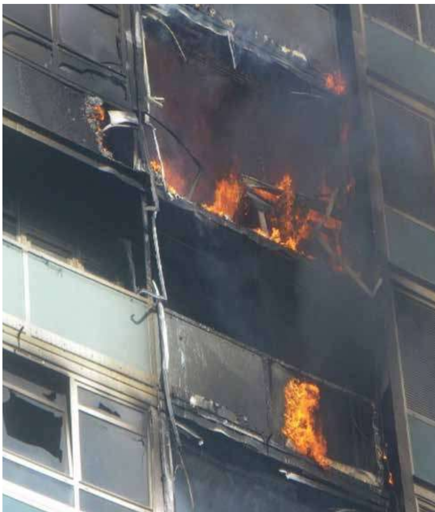
Recommendations of the Lakamal House inquiry in 2013 appear to have been ignored
